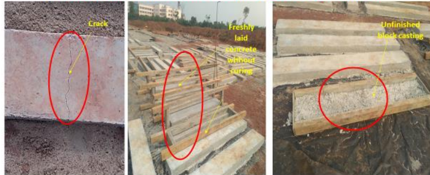
Concrete Paver Blocks have been laid without adequate curing leading to cracks
