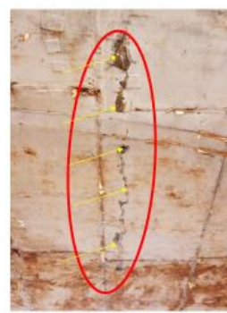
Water dripping from cracked RCC slab: Location - 2
