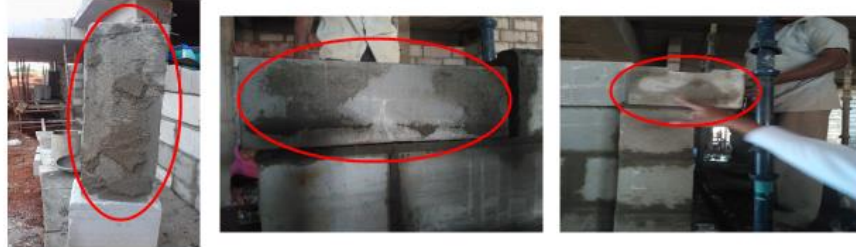
More than 60% of AAC block surface not attached with mortar
