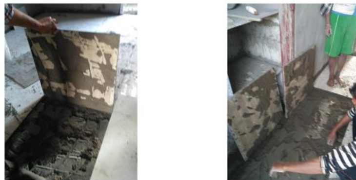
More than 70% of Tile surface not attached with mortar
