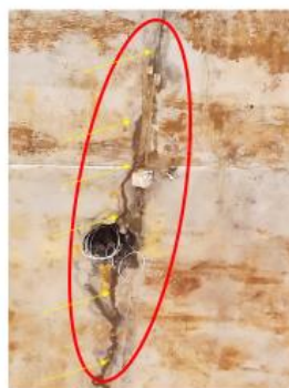
Water dripping from cracked RCC slab: Location - 1
