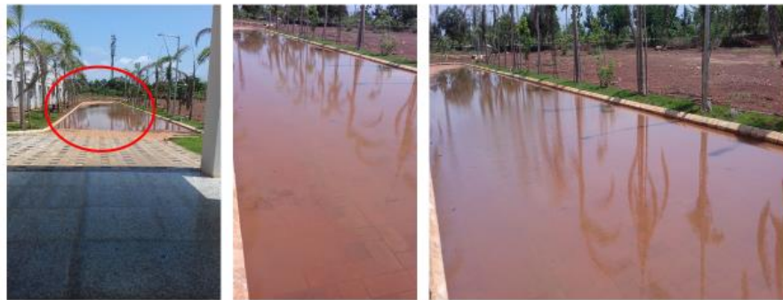
Stagnation of water due to improper slope in pathway
