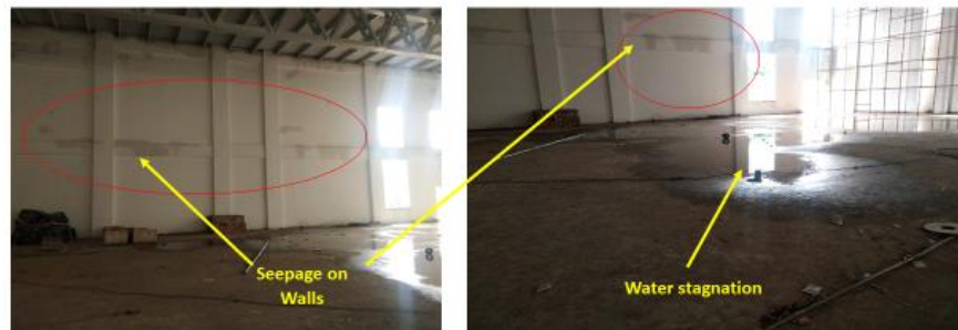
Seepage in the walls are mainly due to poor brick work done by using dry dusty brick, dry cement mortar and poor workmanship
